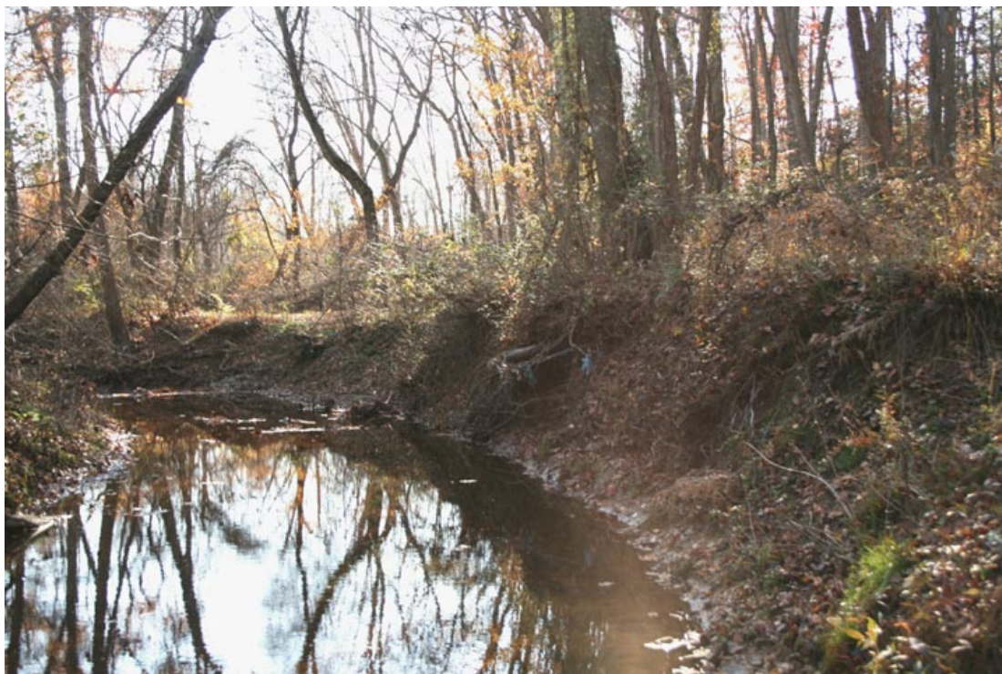
Photo 3.76 – Bank erosion along upper section
