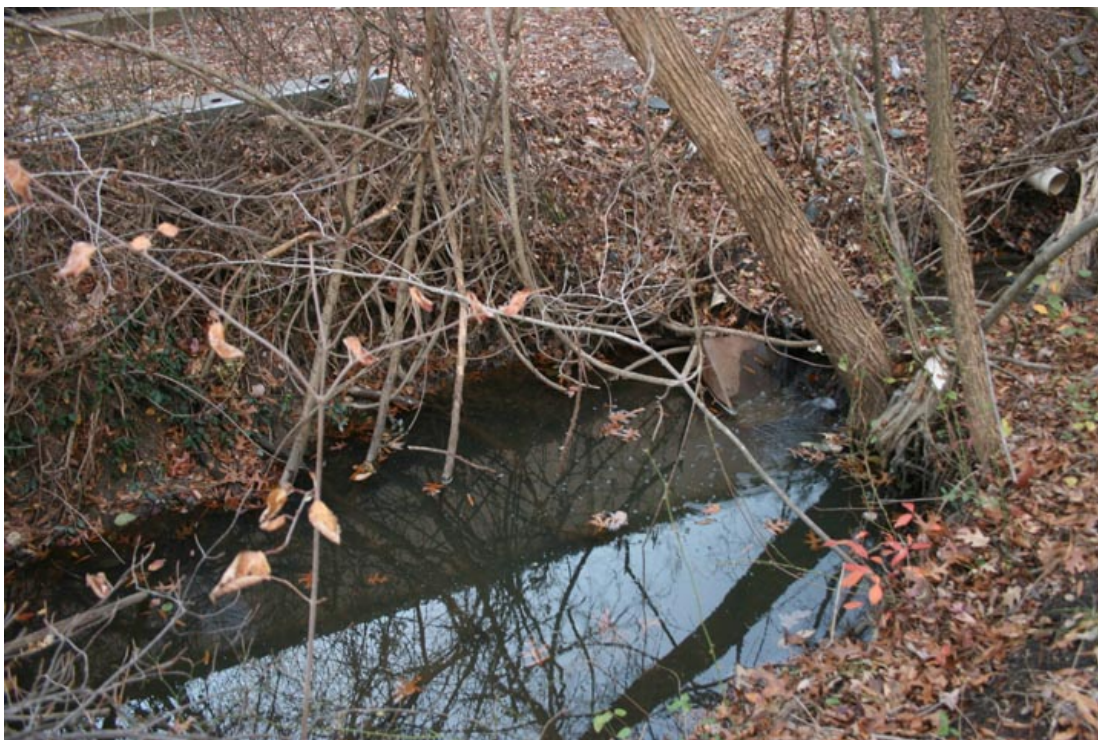
Photo 3.25 – Unstable G4 channel upstream of Route 40
