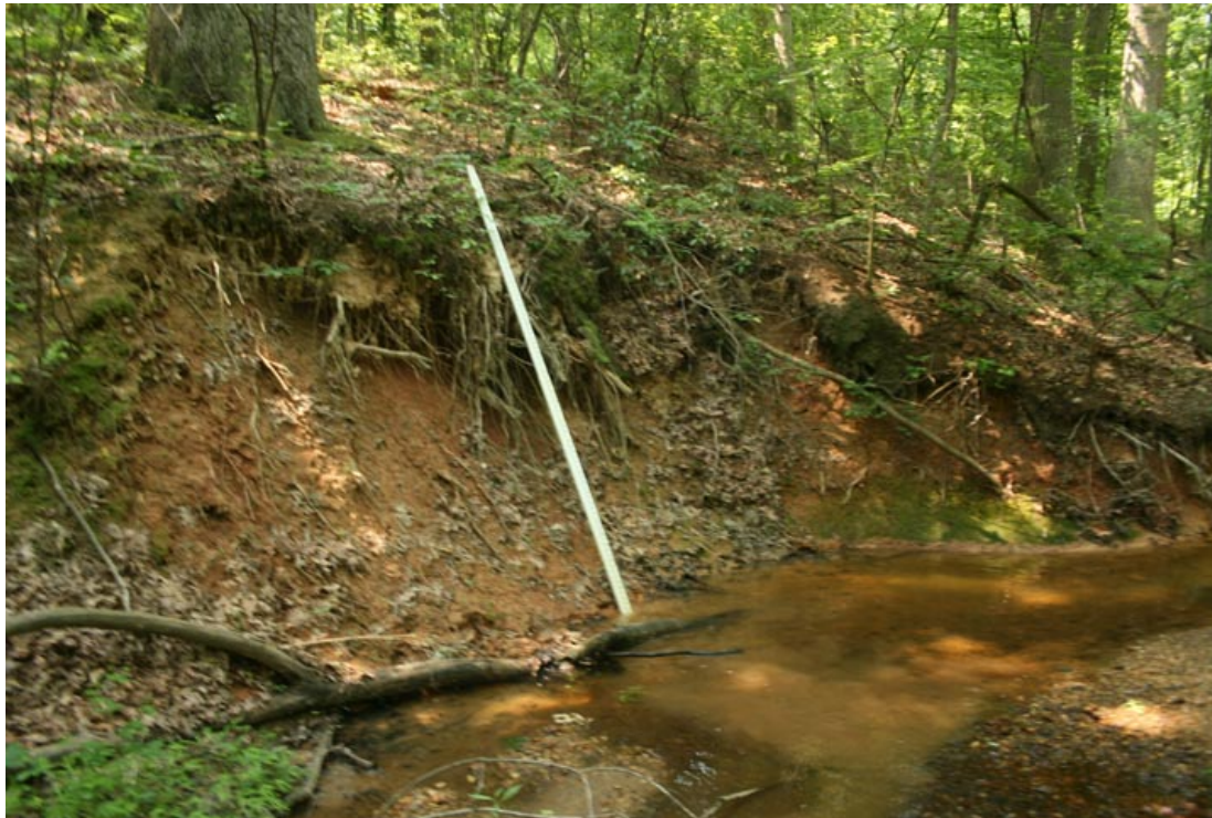
Photo 3.3 – Failing slope along middle section
