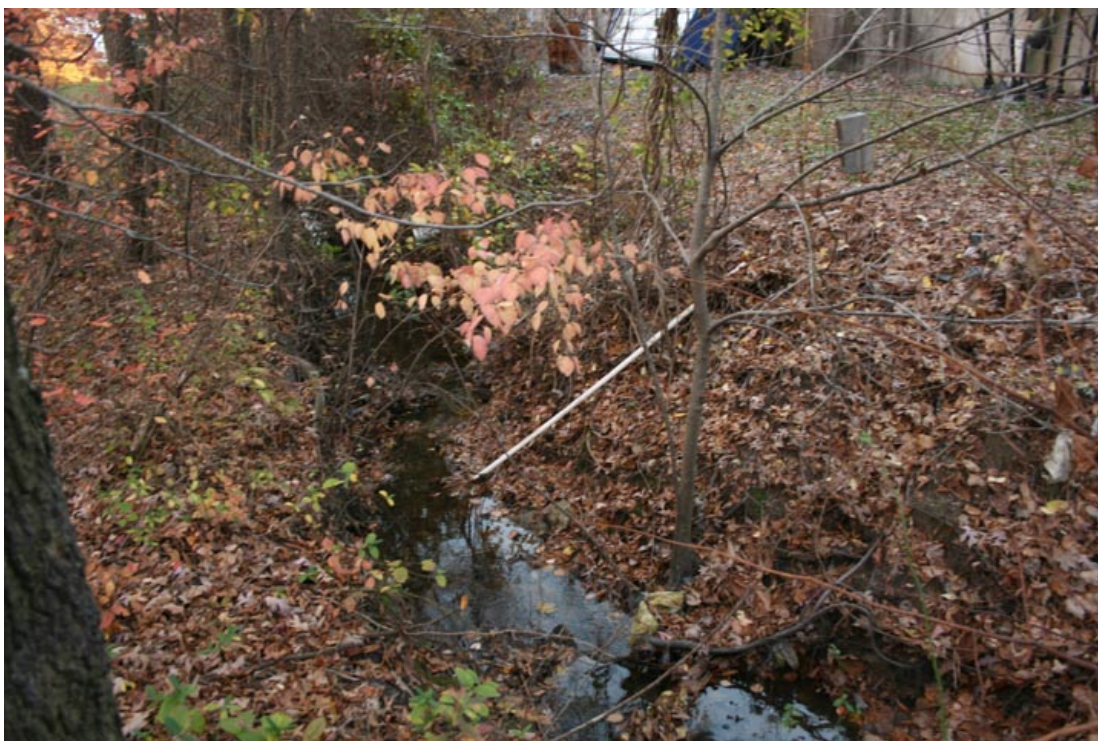
Photo 3.26 – Unstable G4 channel upstream of Route 40
