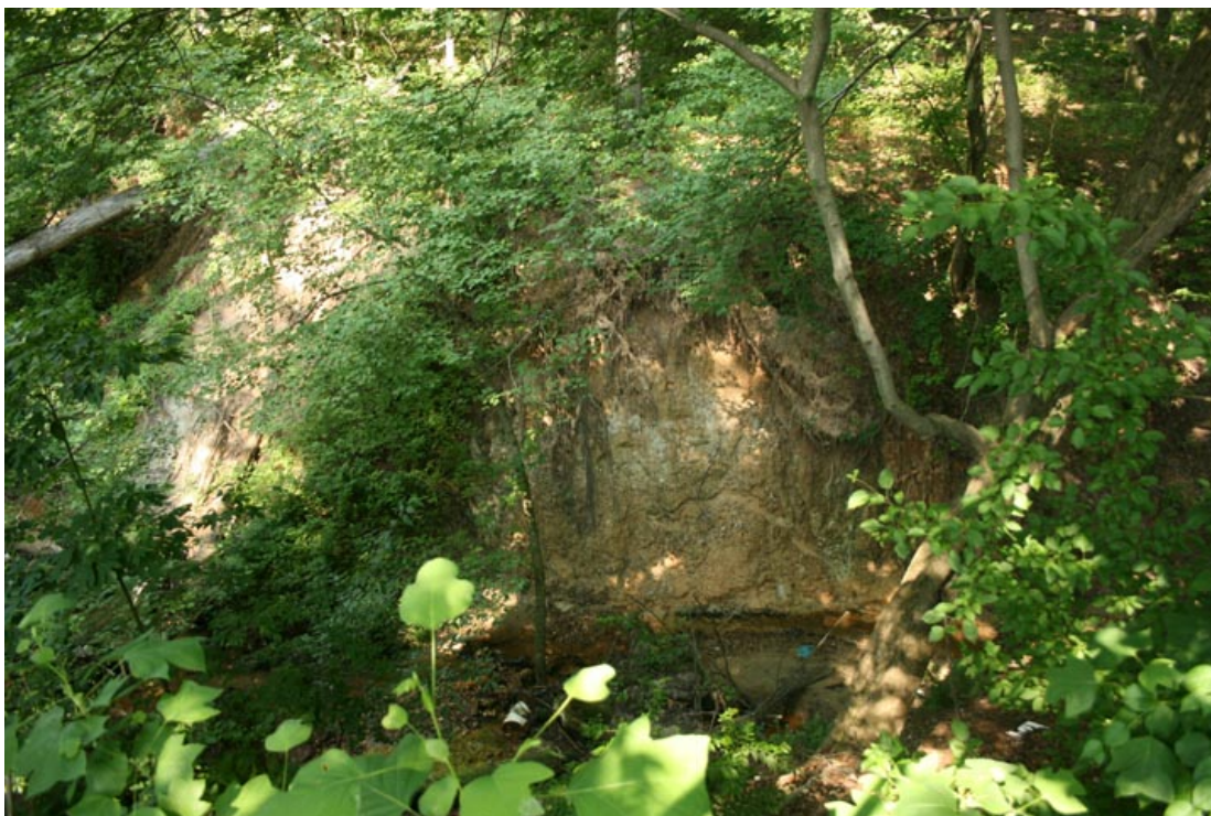
Photo 3.21 – Failing slope along West Tributary
