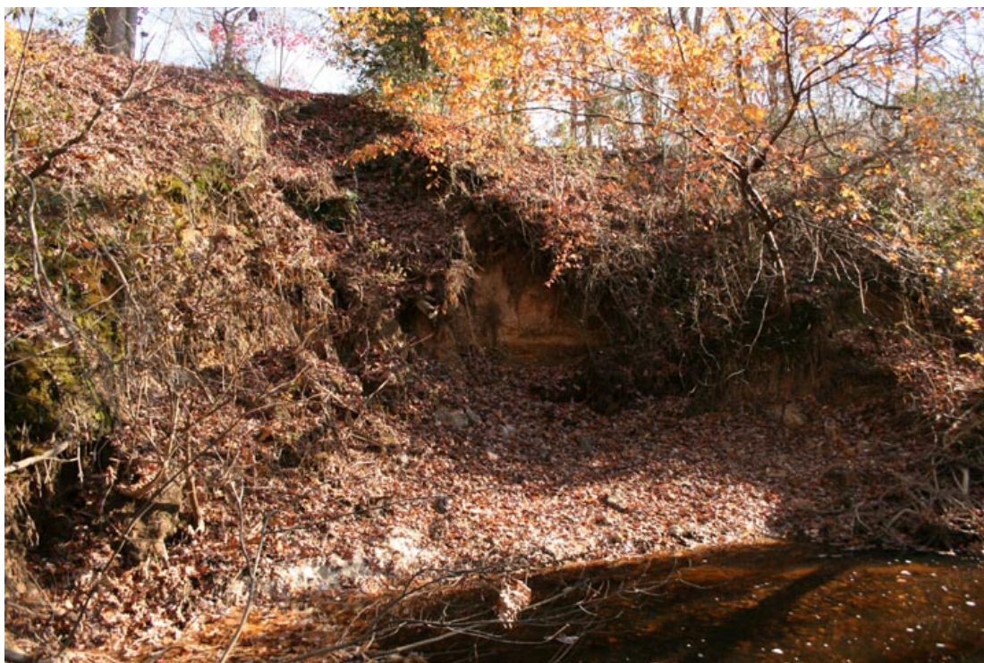
Photo 3.78 – Failing slope along middle section
