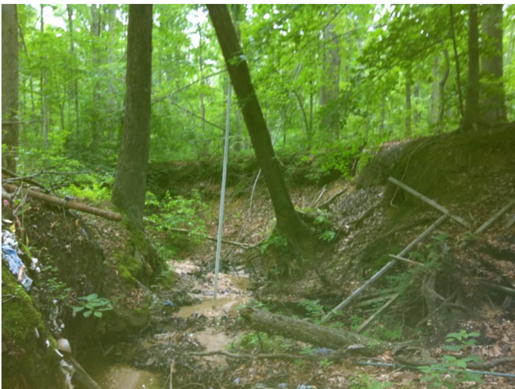
Photo 3.11 – Deeply incised upper section with undercut and falling trees
