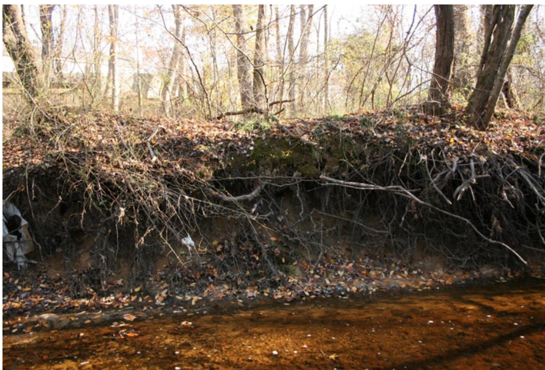
Photo 3.77 – Bank erosion and failing footbridge along upper section
