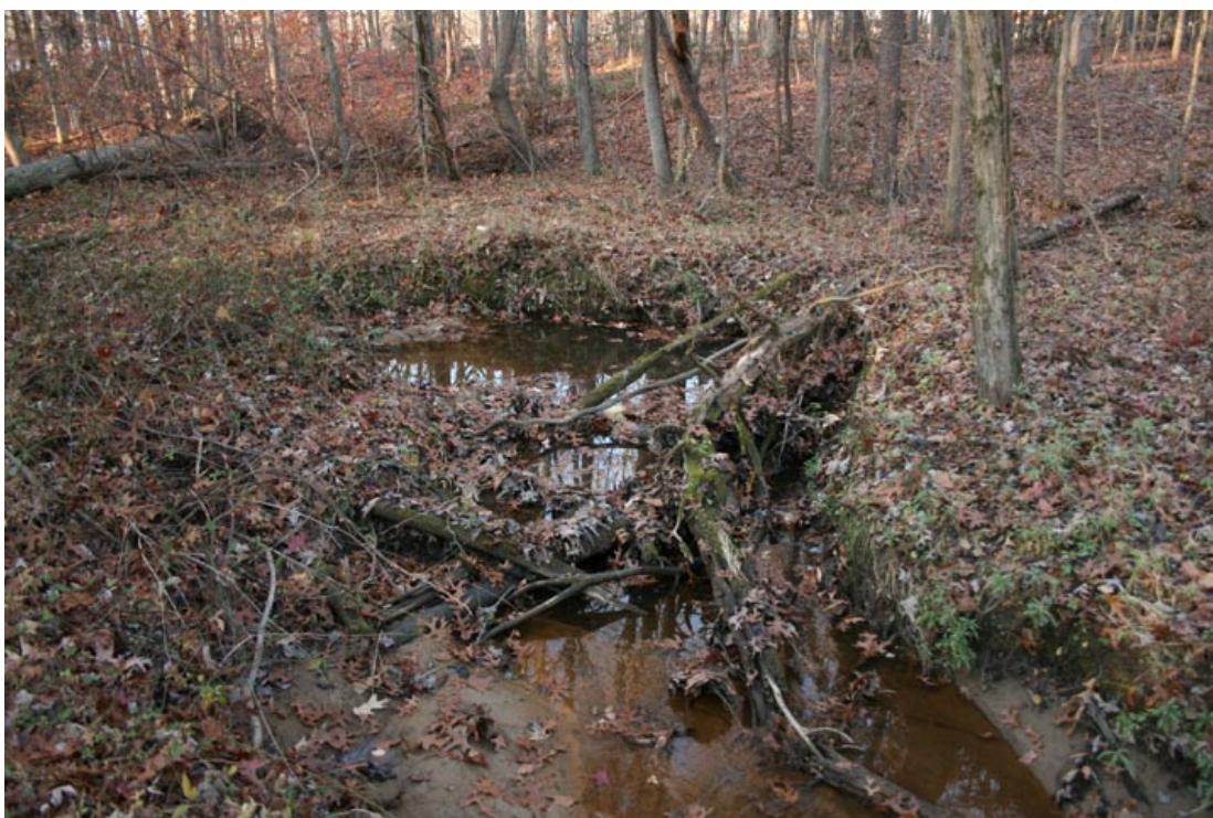
Photo 3.30 – Debris jam along reach downstream of Pine Road
