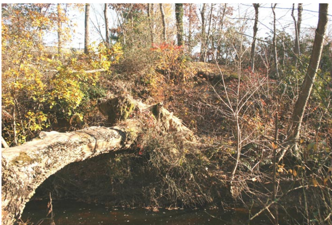
Photo 3.79 – Failing slope along middle section
