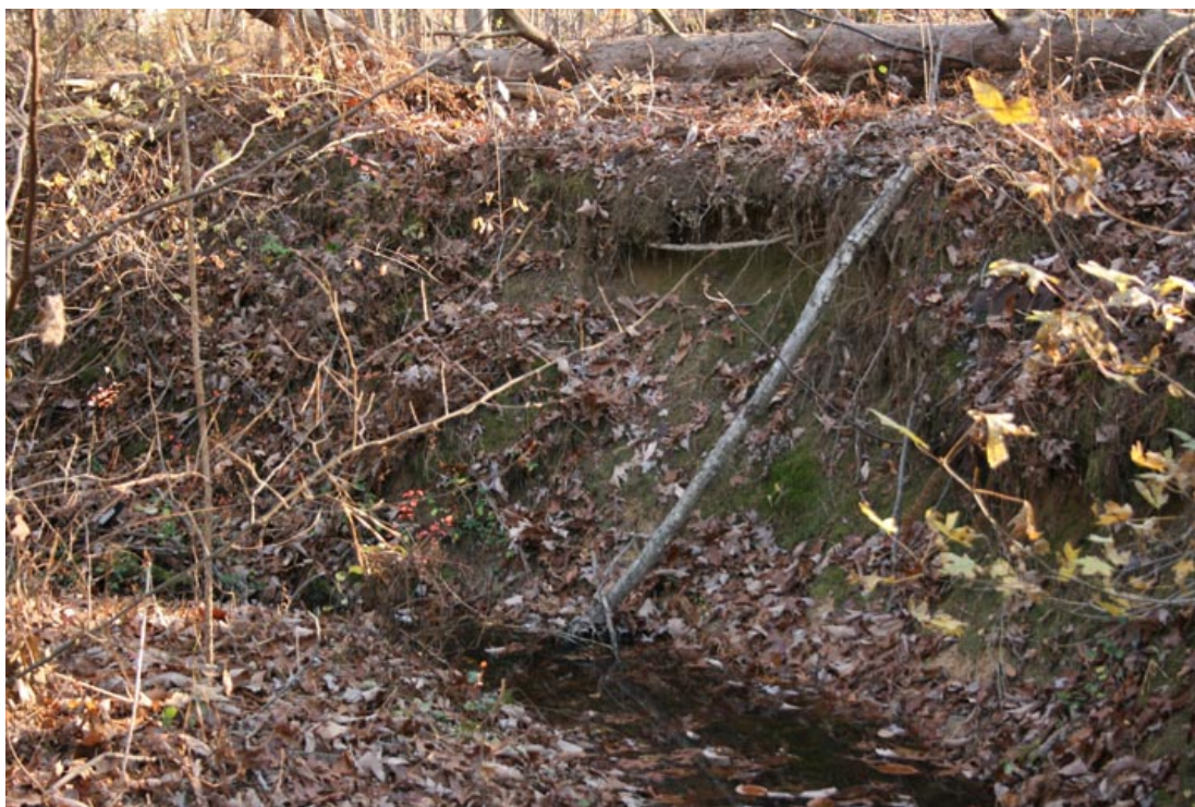
Photo 3.58 – Bank erosion along upper section of South Tributary
