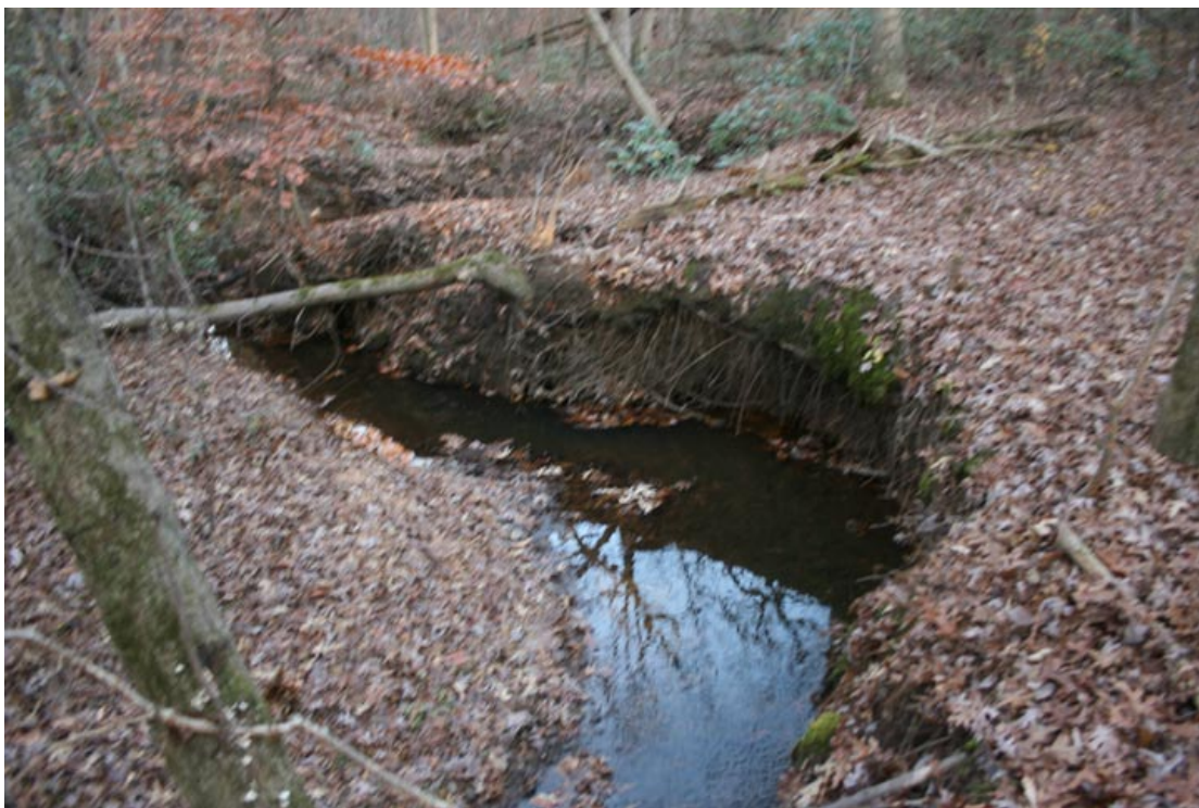
Photo 3.36 – Bank erosion along lower section
