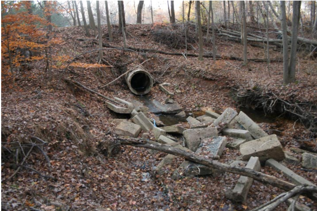
Photo 3.35 – Unstable outfall and channel downstream of pond
