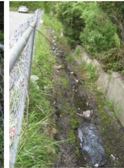
Trash deposition and poor water quality in channel
