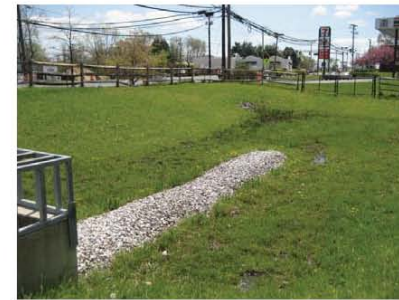
Outflow riser with de-watering device
