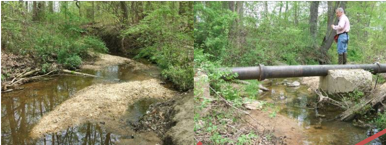
Exposed Pipes in Stream
