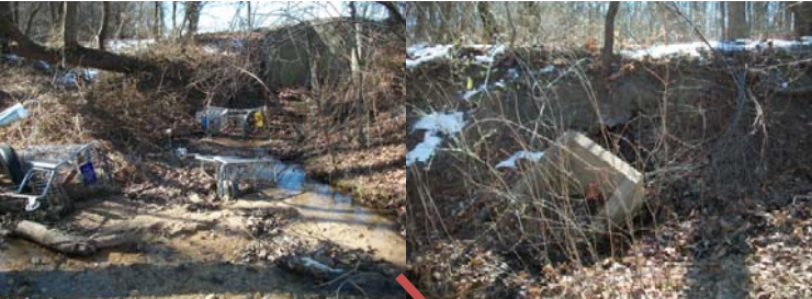
Trash and Debris in Stream, Failed Headwall
