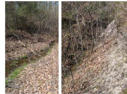
Eroded outfall channel
