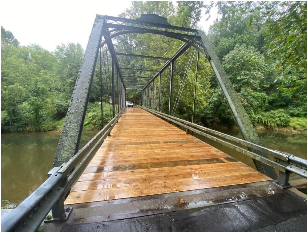
The timber has been replaced on the Cherry Hill Road bridge, which has reopened.
