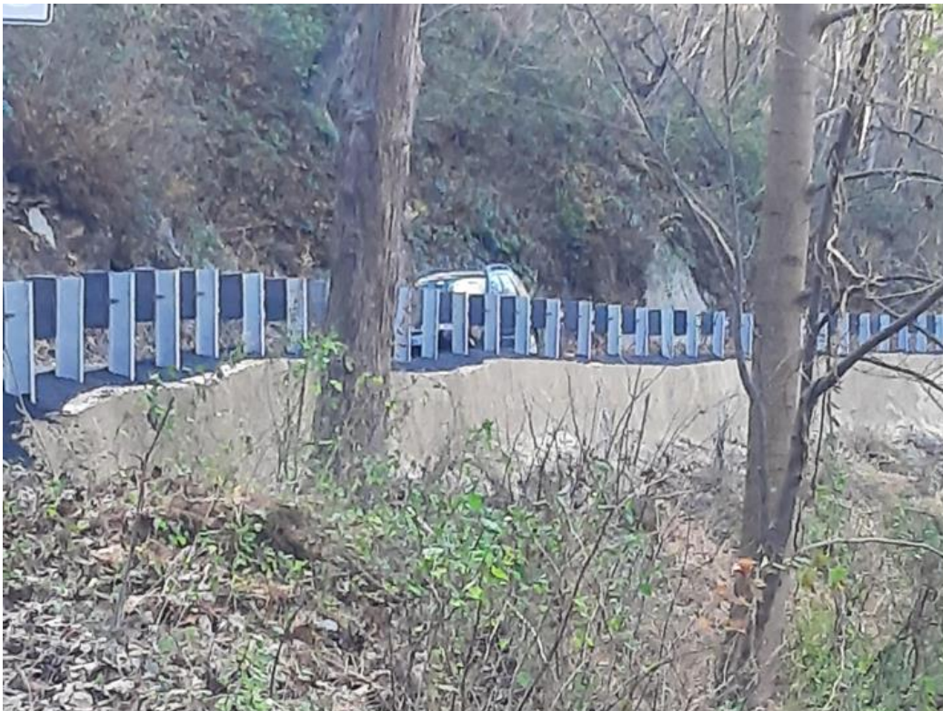
The slope along Madonna Road in Norrisville has been repaired and the road has reopened.
