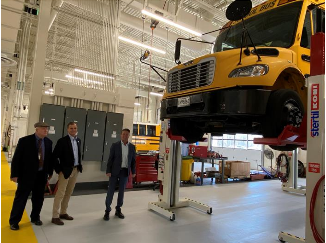
Harford County fleet manager Warren Patrick, advisor to the county executive Billy Boniface, and County Executive Barry Glassman with a school bus raised for repairs.
